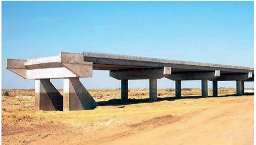
This photograph illustrates a third attempt to construct the Mongu–Kalabo Road in Zambia, after two previous procurements had failed.
